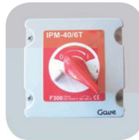
Electrical Isolator fitted to fan for security
